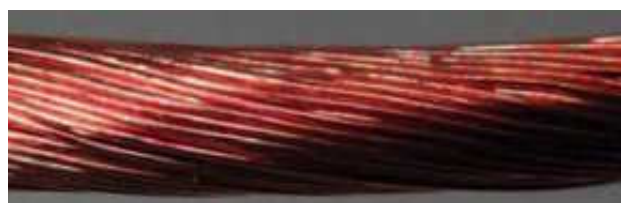
A close-up of the completely intact copper conductor. The inspection performed over the entire length shows that the conductor is still completely intact and does not have any individual wire breakages.
