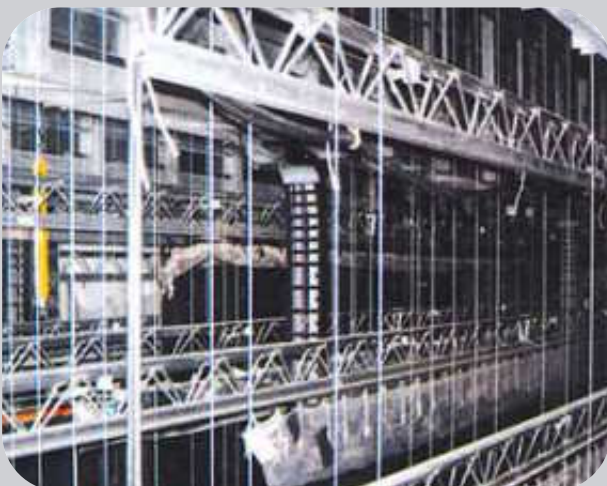
igus® ReadyChain® used for a zigzag application of an illumination cross arm, Royal Opera, London
